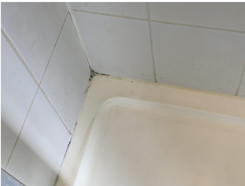
Localised mould growth at a tile and sealant junction, typically associated with high humidity and restricted airflow.
