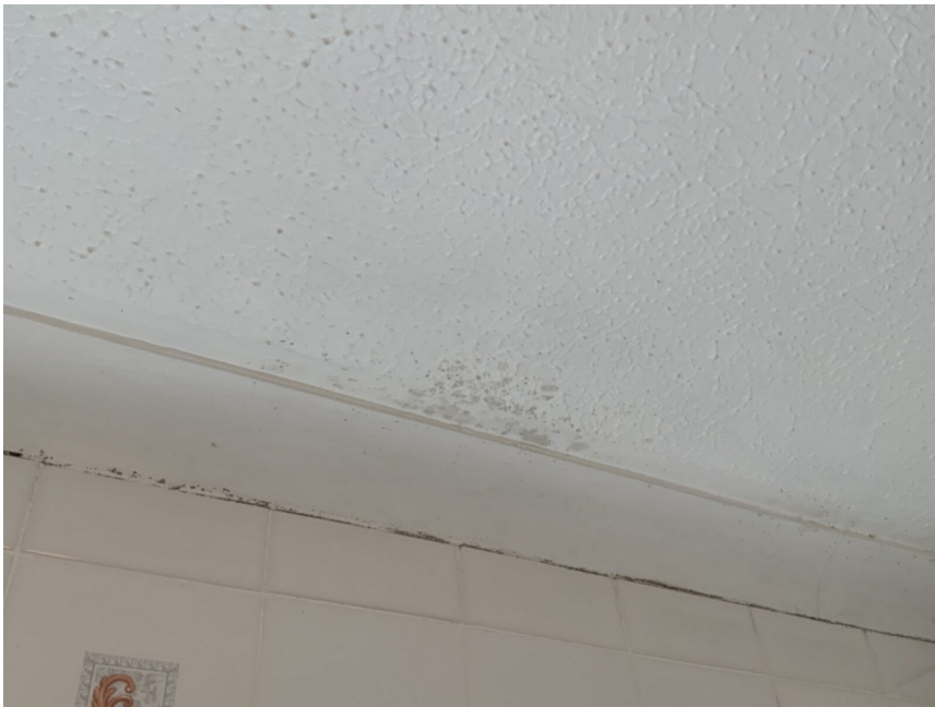
Typical condensation-related mould forming to a ceiling where warm, moisture-laden air meets a colder surface.
