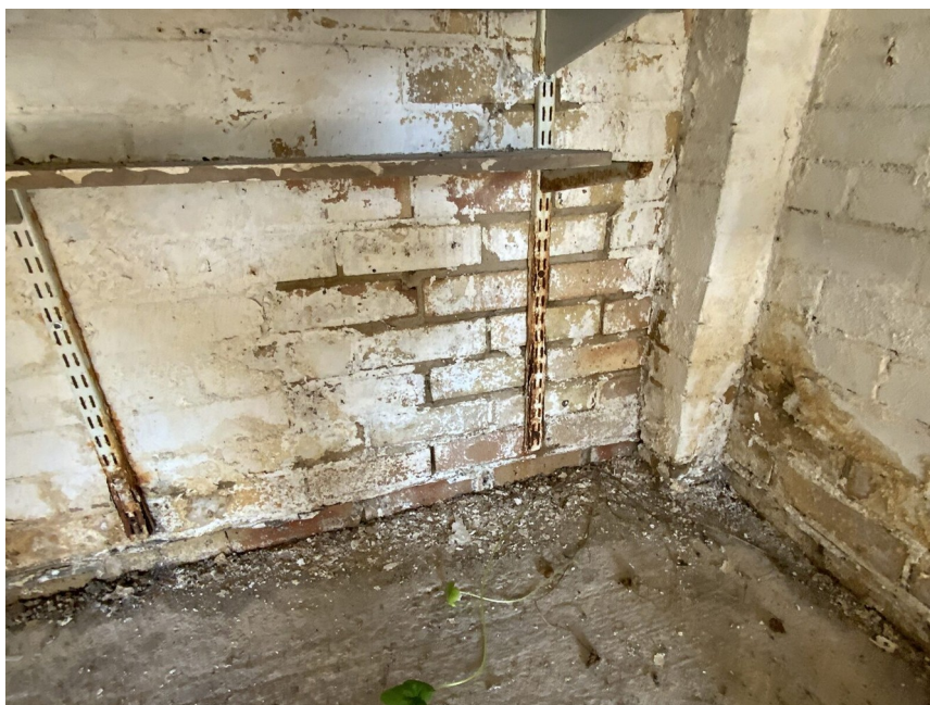
Penetrating damp with associated salt contamination indicating moisture ingress through the building fabric rather than condensation.
