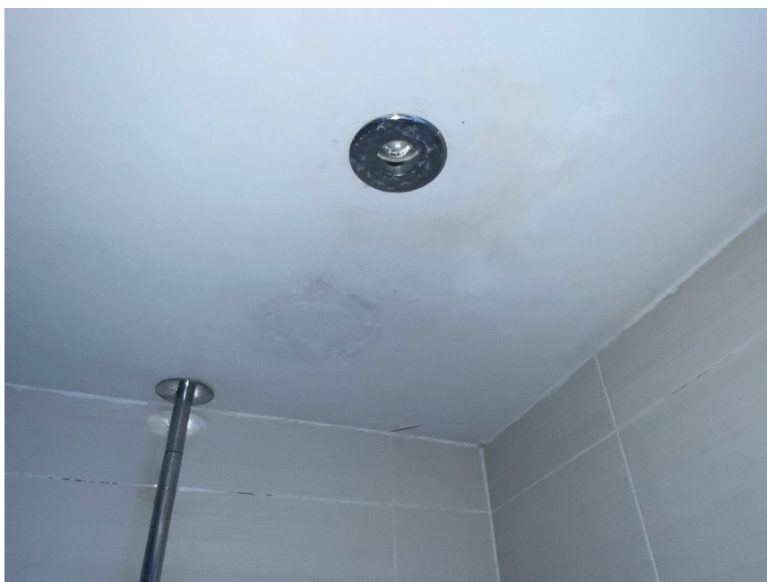
Condensation staining above a shower where moisture is not adequately removed, typically due to missing or ineffective extraction.
