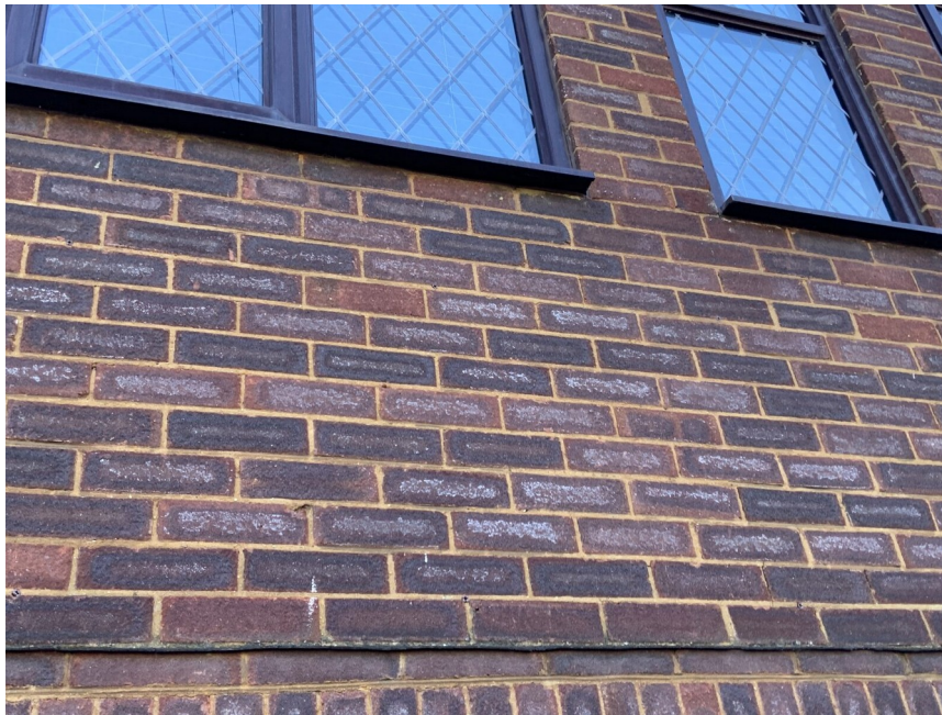
External efflorescence to brickwork showing salts deposited as moisture evaporates from the masonry.
