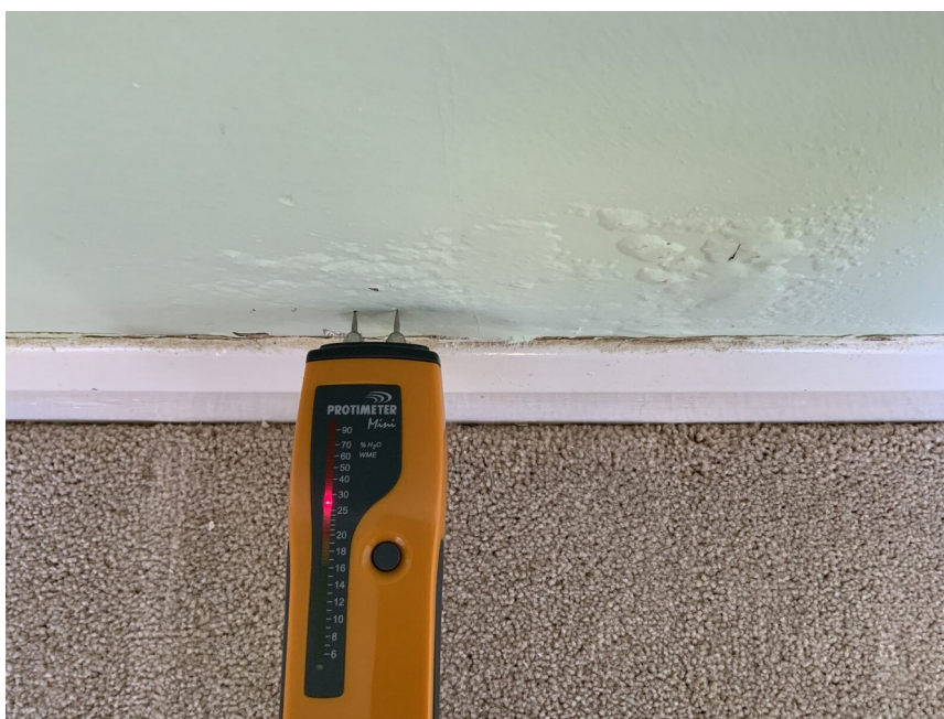
Moisture meter reading indicating elevated dampness within building fabric, used to distinguish between condensation and structural moisture.
